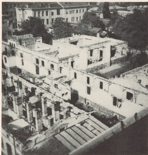
FIGURE 66. Damage to Surgical Clinic, University of Leipzig, by air raid of 4 December, 1943.
