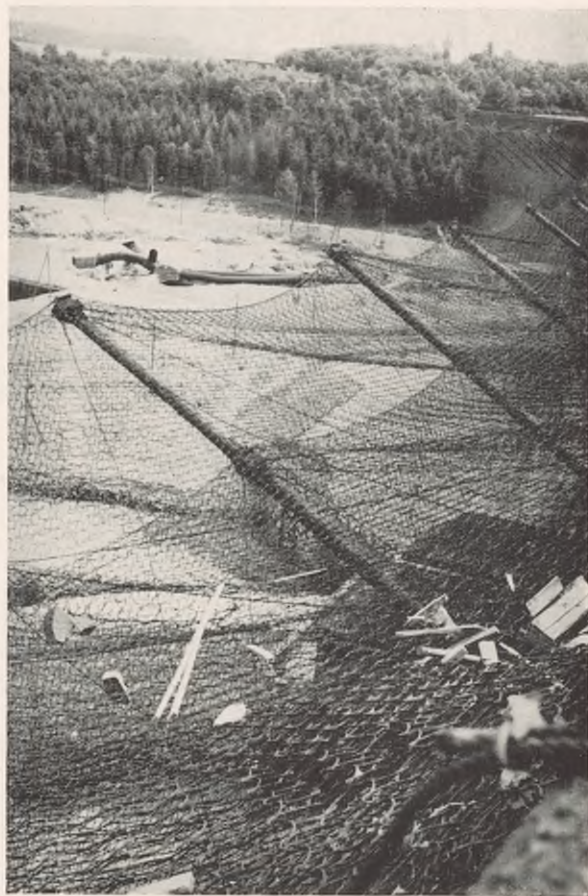
FIGURE 139. Moehne Dam—Steel nets installed on the downstream side, after reconstruction, to prevent bombs dropped vertically from reaching base of dam.
