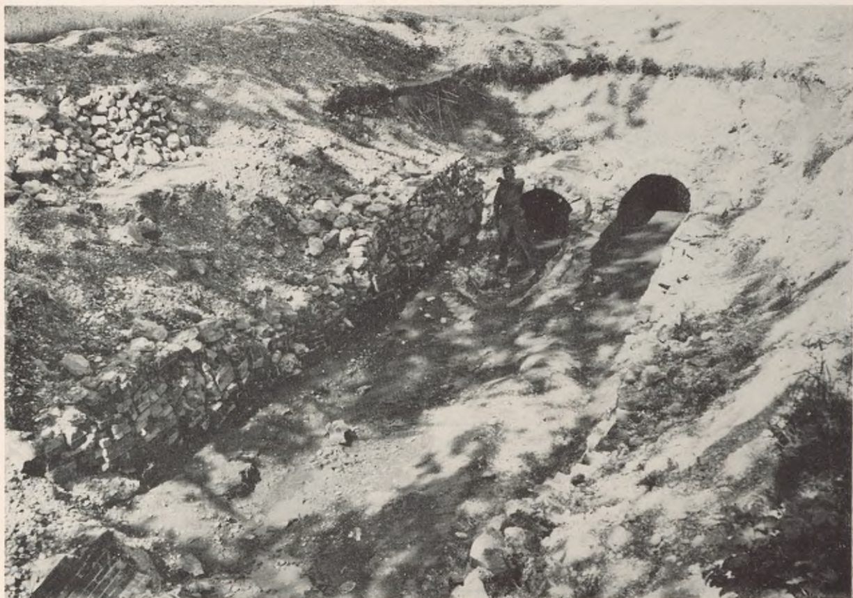
FIGURE 142. Damage caused by direct bomb hit on trunk sewer during air raid—Munich.
