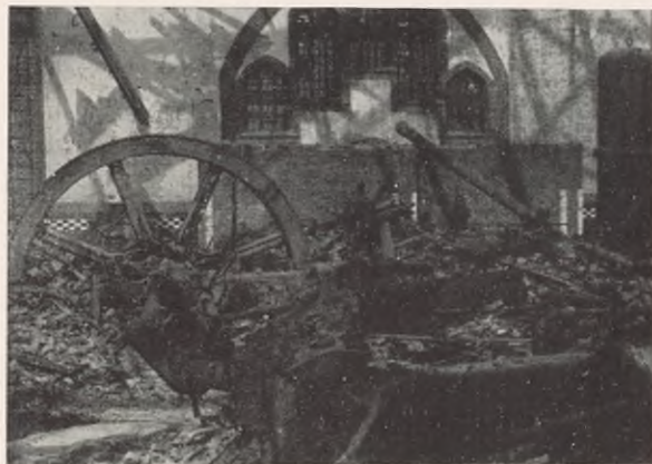
FIGURE 124. Wreckage of pump station—Cologne. Direct hit during air raid.
