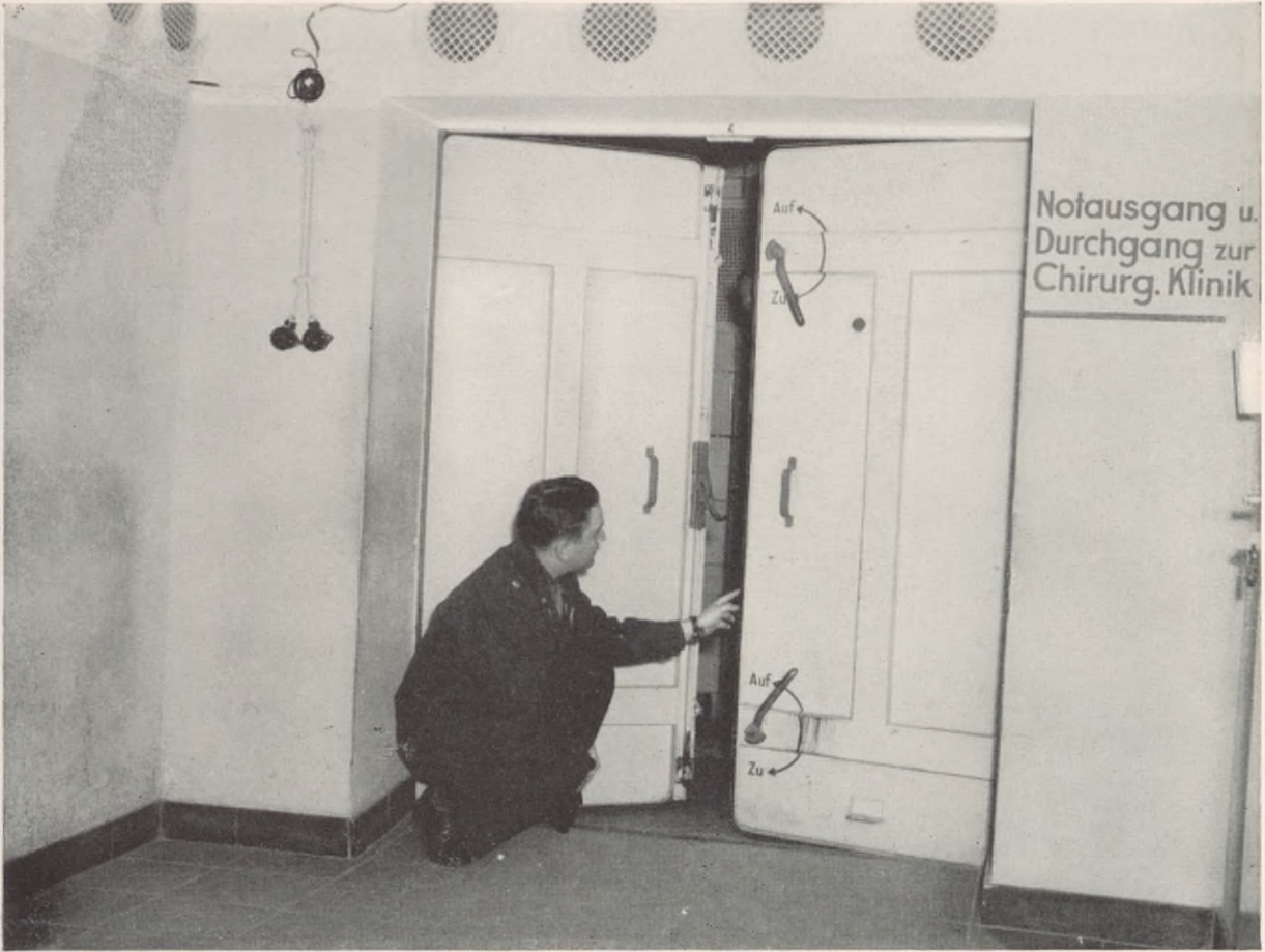
FIGURE 75. Air raid hospital bunker. (Concrete air raid shelter). Gas lock in entrance hall to wards. Note ventilation openings above the door and electrical wiring on the wall. German sign on the right indicates that doorway is an emergency exit, and a passage to the surgical clinic.
