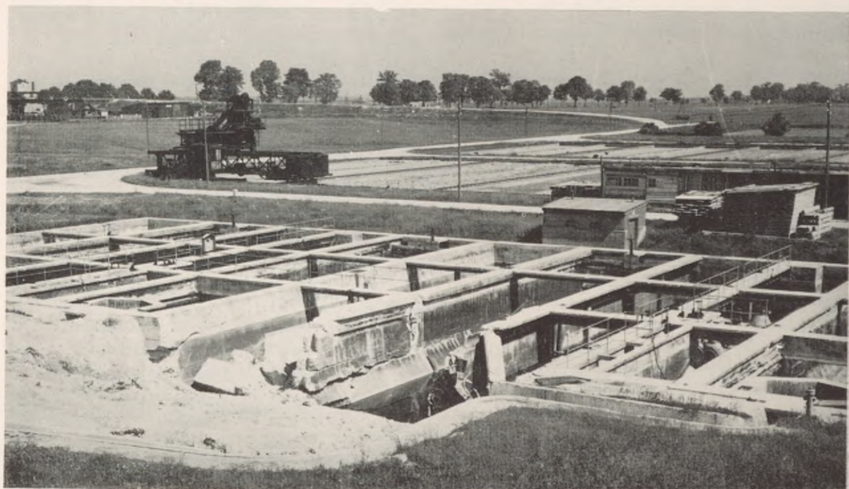
FIGURE 143. Bomb damaged settling tanks—Munich sewage disposal plant. Sludge drying beds in rear.
