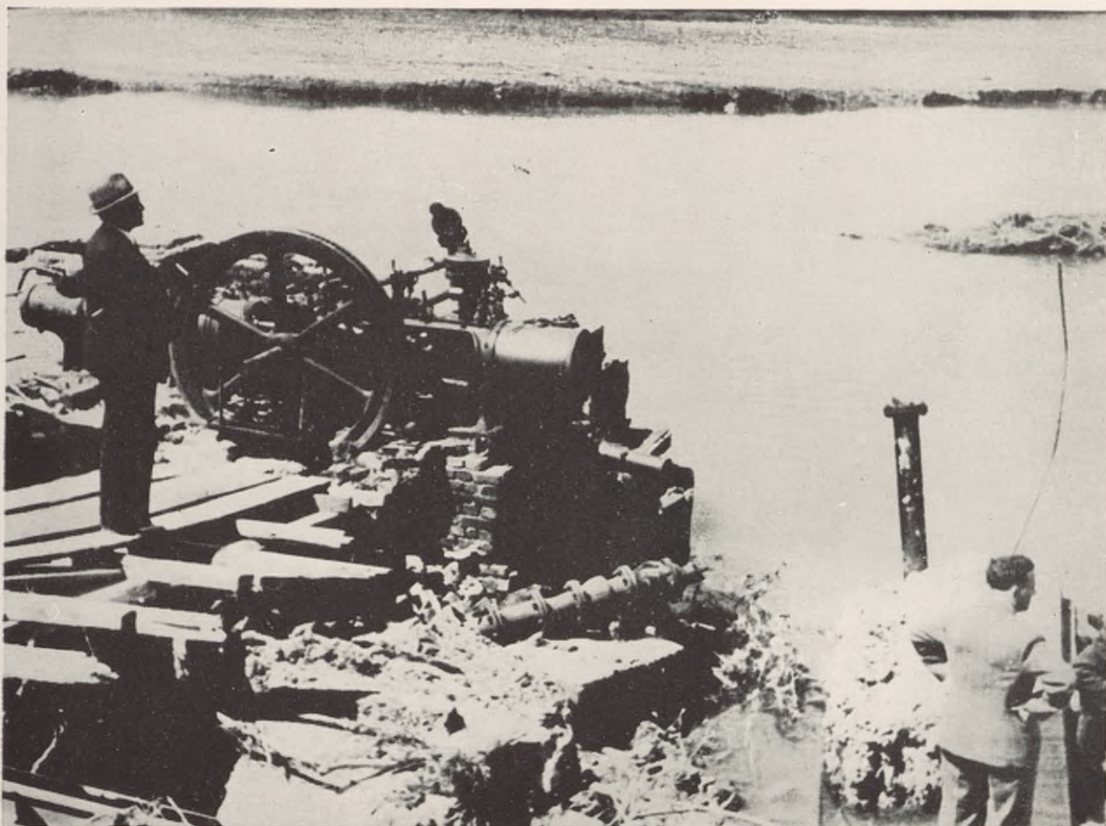
FIGURE 135. Pumping equipment damaged by flood—Neheim water works, May, 1943.
