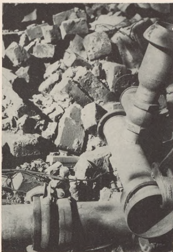
FIGURE 118. Emergency water line—spare stub and valve used by repair team following an air raid. Note quick coupling device—annular rubber gasket used between sections. Line withstands a pressure of 150 pounds per square inch.
