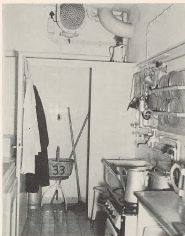
FIGURE 92. Air raid hospital bunker, Frankfurt on Main, typical compact diet kitchen. Note exterior installation of electrical facilities, and water and sewer pipes. Small general utilities closet in rear. Electrical stove on the right. Electrical refrigerator on the left.
