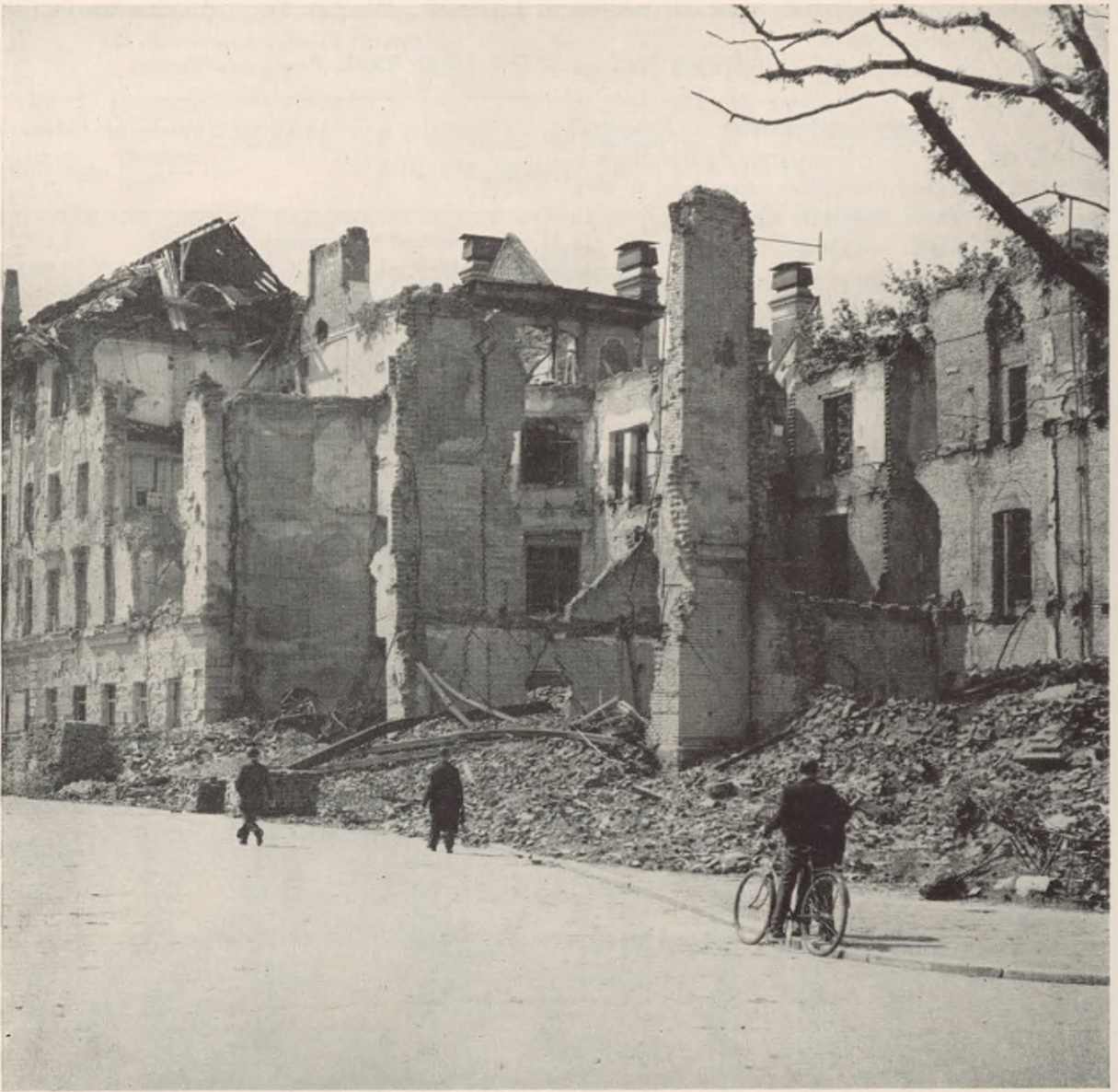
FIGURE 57. Air raid damage to First Medical Clinic, University of Munich. Front view.
