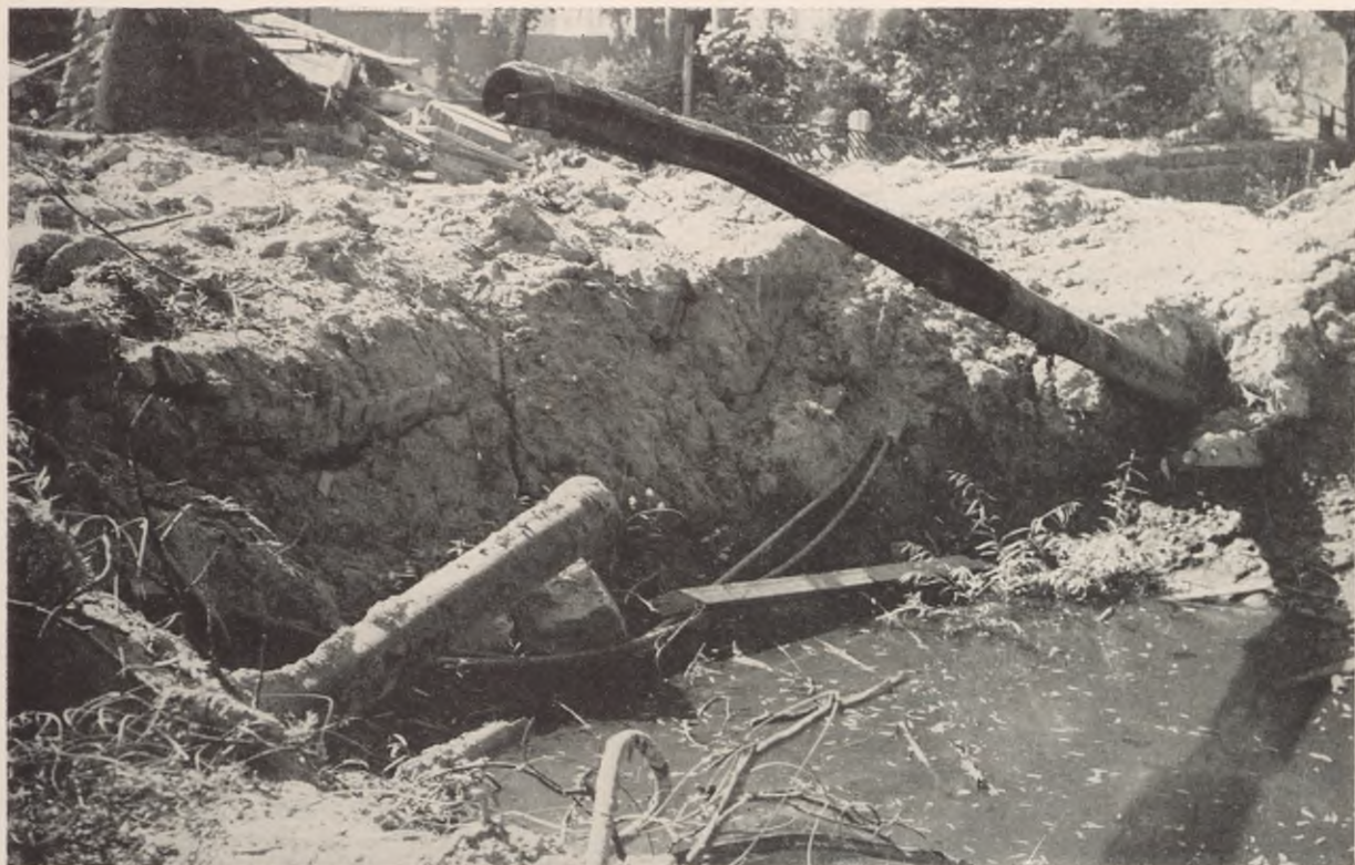
FIGURE 131. Typical damaged (8") steel water line. Note distortion. Result of direct bomb hit during air raid.
