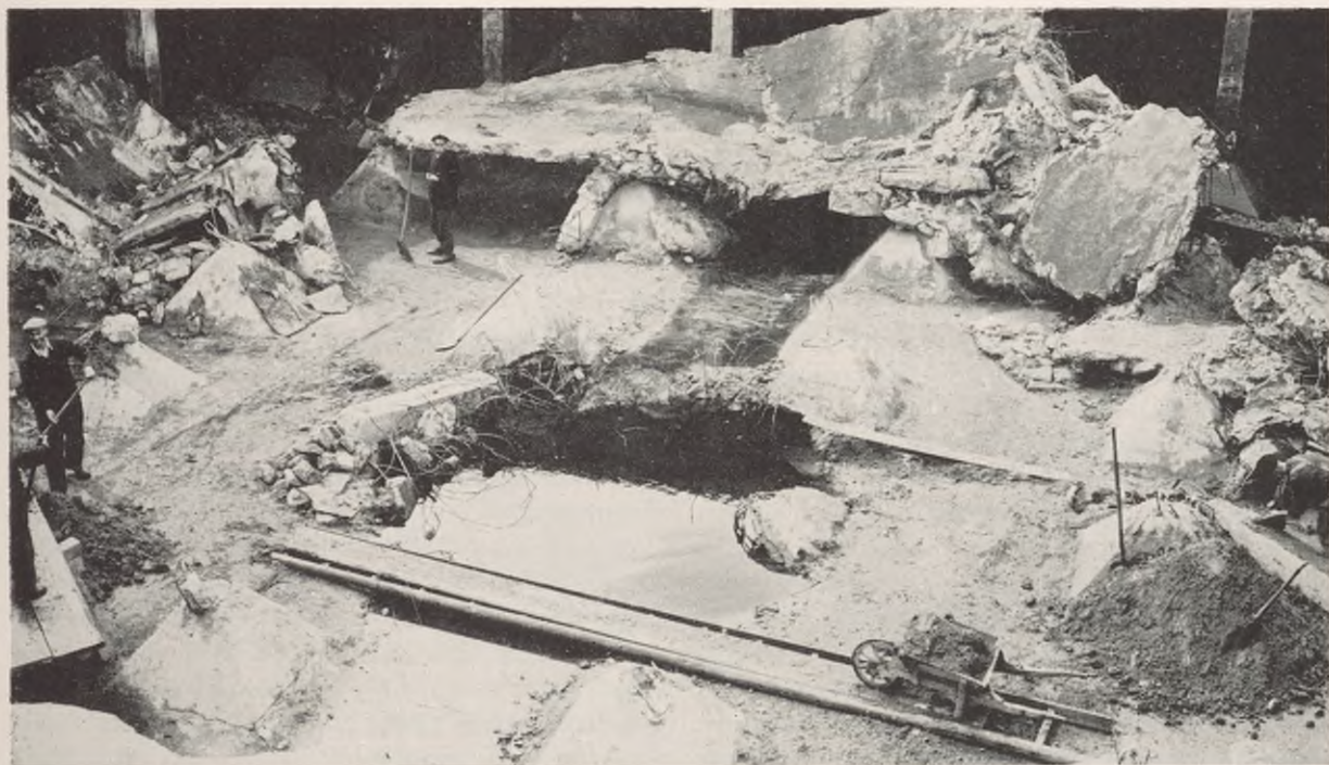
FIGURE 129. Bomb damaged reservoir (5 million gallons capacity)—Hamburg.
