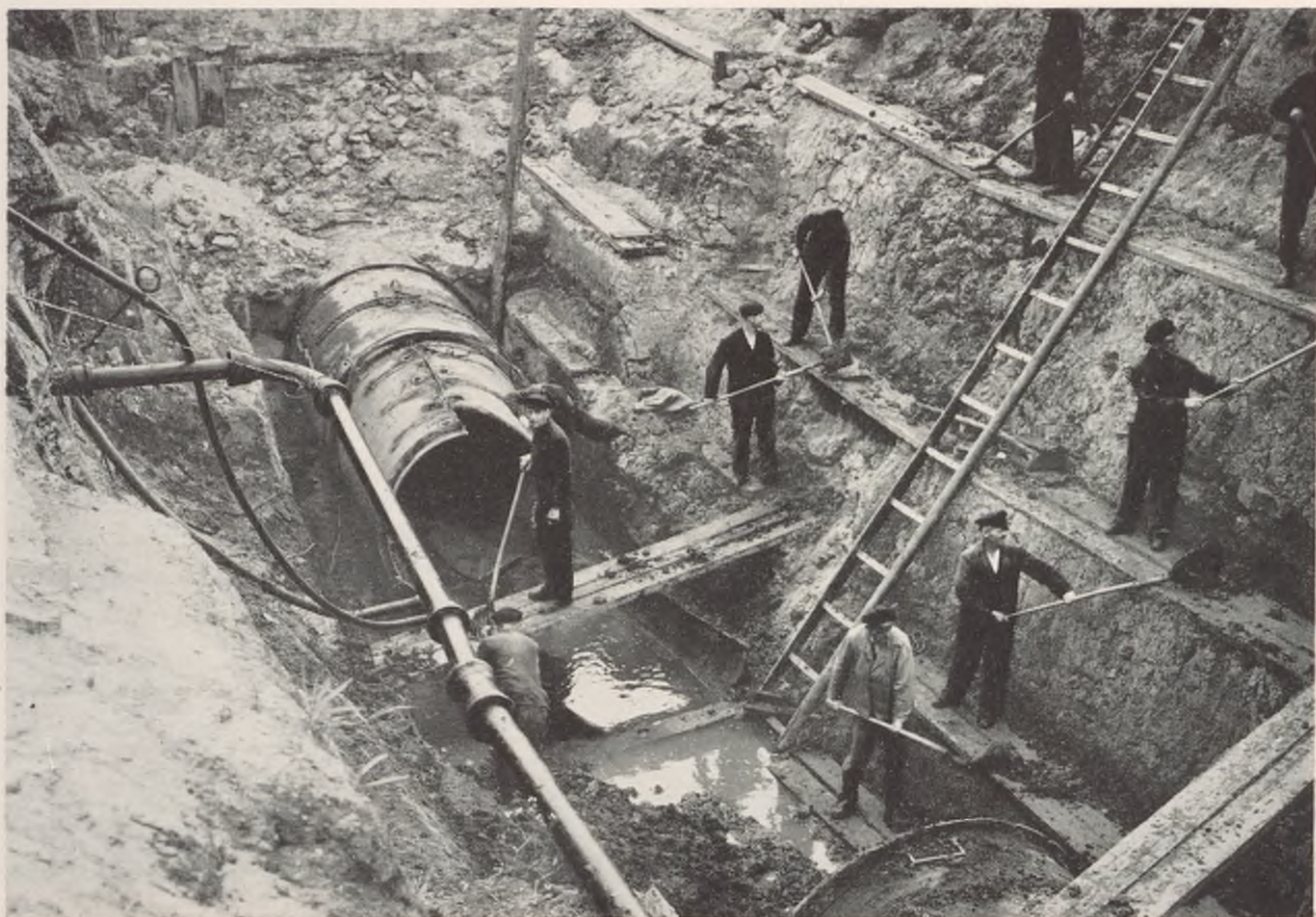
FIGURE 128. Broken suction line (80" diameter) at Hamburg pumping station.
