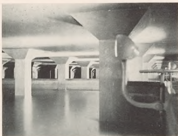
FIGURE 122. Interior of underground water reservoir—Munich. Capacity—185 million gallons. Covered with artificial landscaping to conceal its location and identity.
