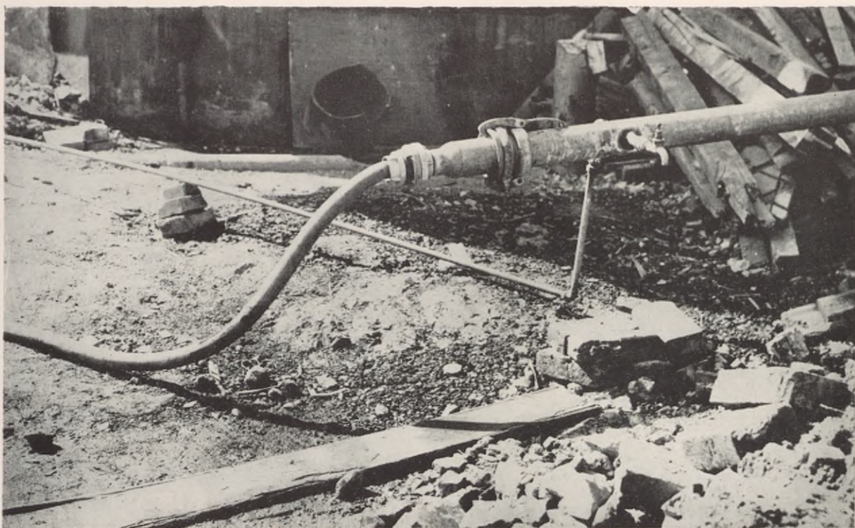
FIGURE 116. Emergency pipe line laid on air raid rubble, with hose connection and branch pipe. Note faucet welded directly into pipe.
